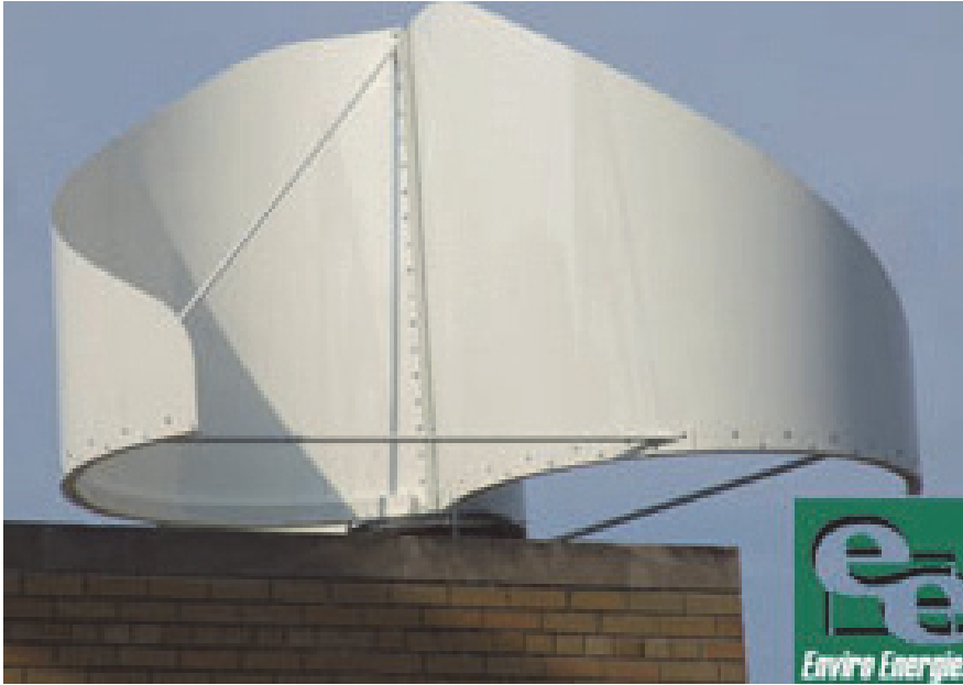
Fig. 2. VAWT made by Enviro-Energies and installed on the company's roof
